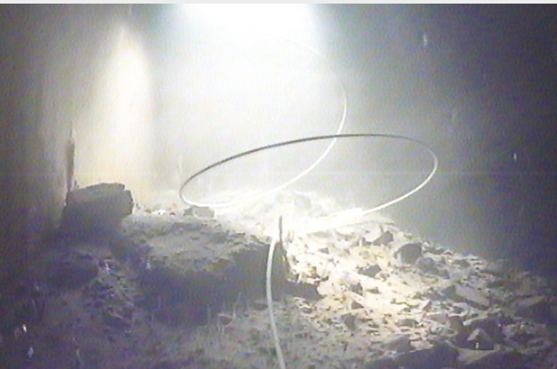
Video images of debris in the tank from the on-board video camera
