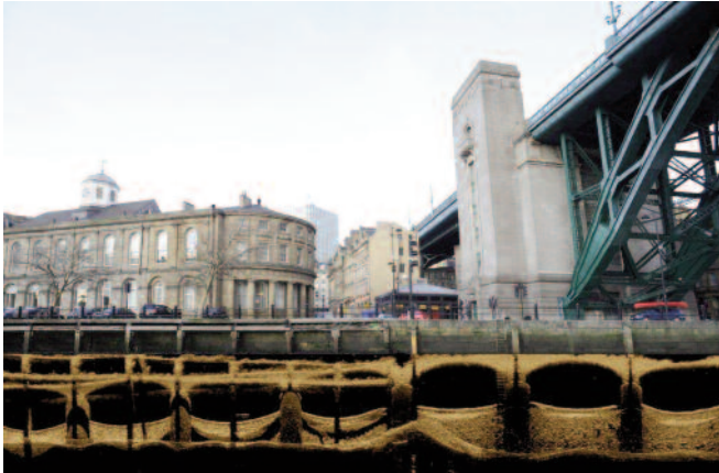
Image of Tyne River harbour wall, the overlaid sonar image below clearly shows the wall supports
